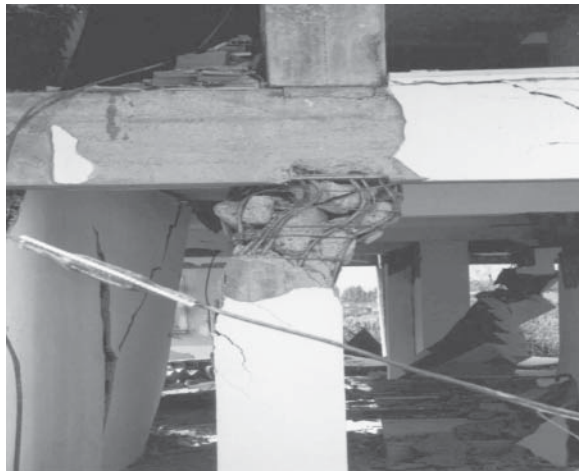
Lack of transverse reinforcement. Courtesy of Murat Saatcioglu and John Gardner
