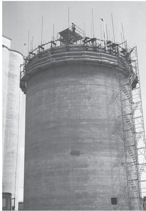
Reinforced concrete grain silo using the slip form system. Brookings, South Dakota.
