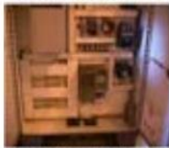
Electric Drive Control Unit
