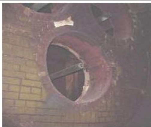
Figure 1.3 Burner end of sulfur burning furnace. Atomized molten sulfur droplets are injected into the furnace through steam-cooled lances. Dry combustion air is blown in through the circular openings behind. The sulfur is oxidized to SO 2 by Reactions (3.1) and (3.2). Atomization is done by spiral or right angle flow at the burner tip.
