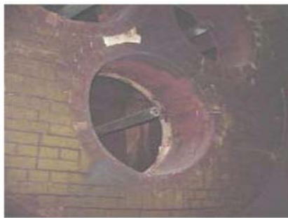
Figure 3.3 Burner end of sulfur burning furnace. Atomized molten sulfur droplets are injected into the furnace through steam-cooled lances. Dry combustion air is blown in through the circular openings behind. The sulfur is oxidized to SO 2 by Reactions (3.1) and (3.2). Atomization is done by spiral or right angle flow at the burner tip.
