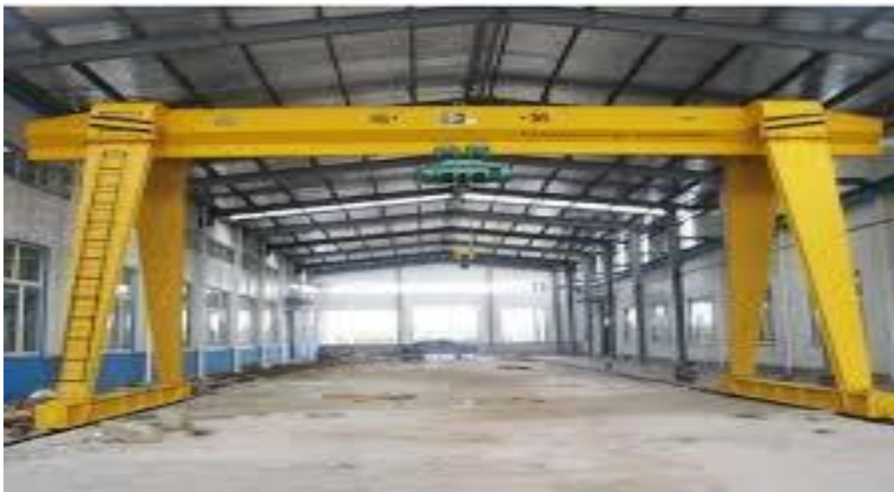
1.7 Rasm Ishlab chiqarish binosi ichidagi chorpoyali kran
